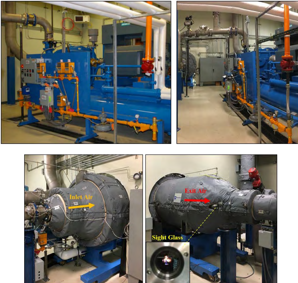
Figure 2-10. Natural Gas Delivery System Installed at START During 2016 and the Combustion-based Heater Chamber. Image credit: PSU
