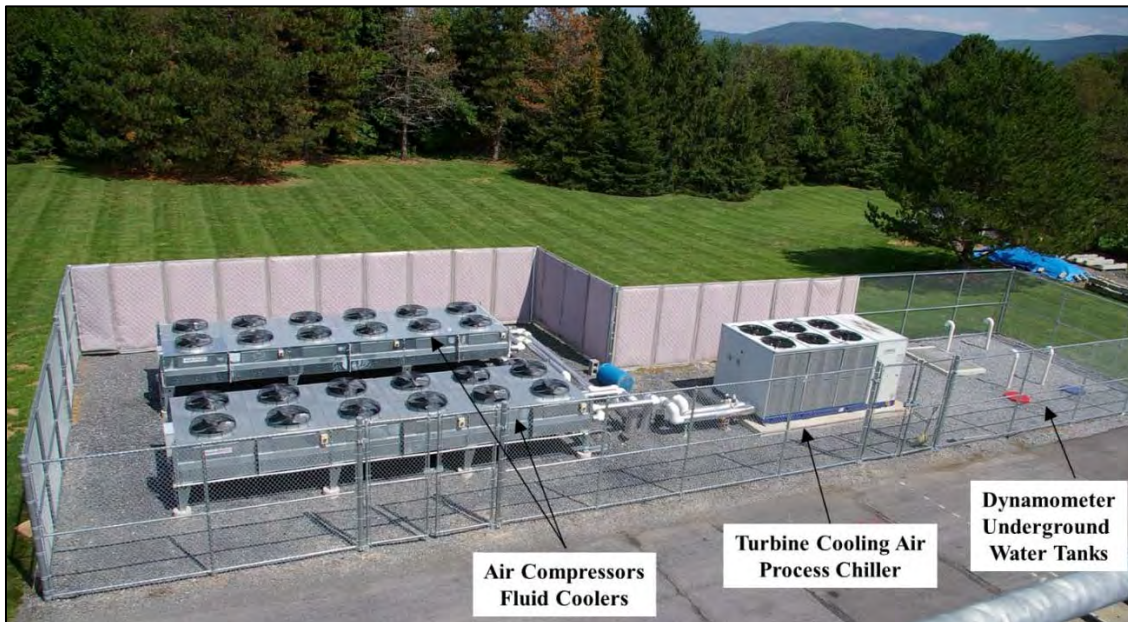
Figure 2-9. Outdoor Large Cooling Systems for the Compressors and Test Turbines, Including an Underground Water Tank System, Installed for the START Facility During 2013-2016. Image credit: PSU
