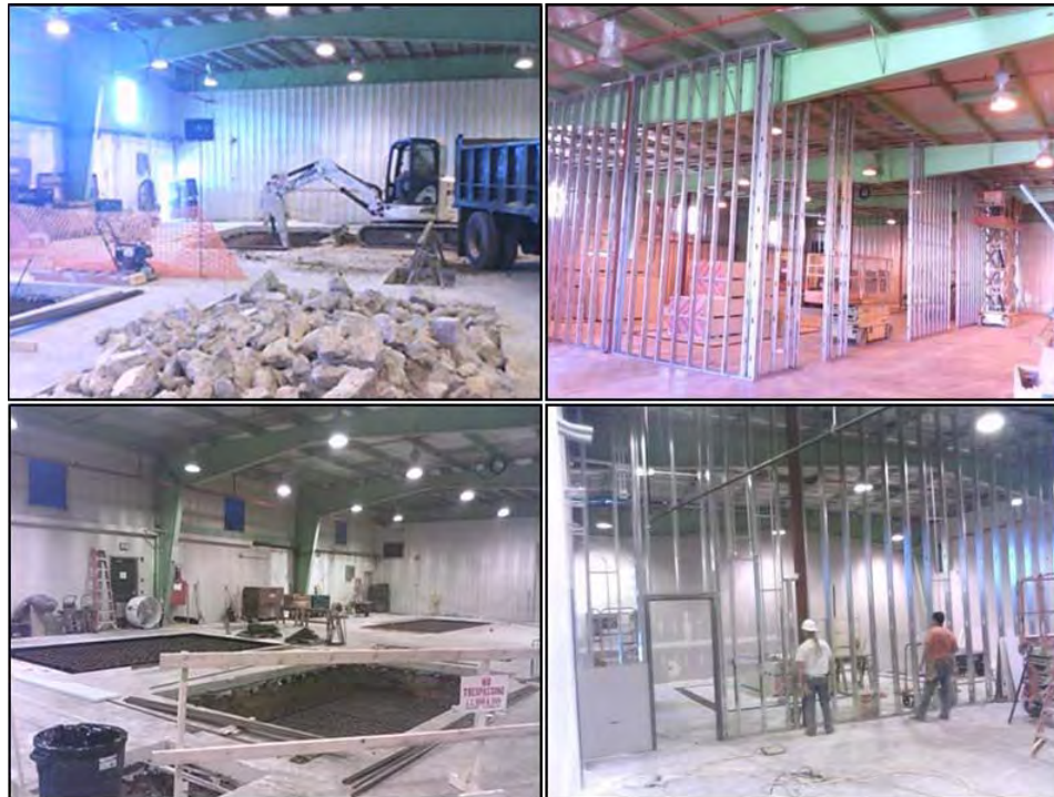
Figure 2-4. Renovation and Construction Work Performed at the START Facility Building in 2012 Within the Large High-bay Room. Image credit: PSU
