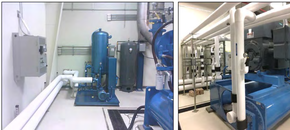
Figure 2-8. Indoor Circulation System for the Air Compressor Cooling Fluid Installed for the START Facility During 2013-2016. Image credit: PSU
