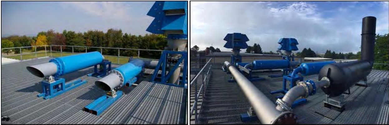
Figure 2-11. Outdoor Roof Platform Installed Above the START Facility Compressor Room. Image credit: PSU Including the air flow intake systems and turbine exhaust silencers for a single air compressor operation in 2014 (left) and for dual air compressor operation in 2016 (right)
